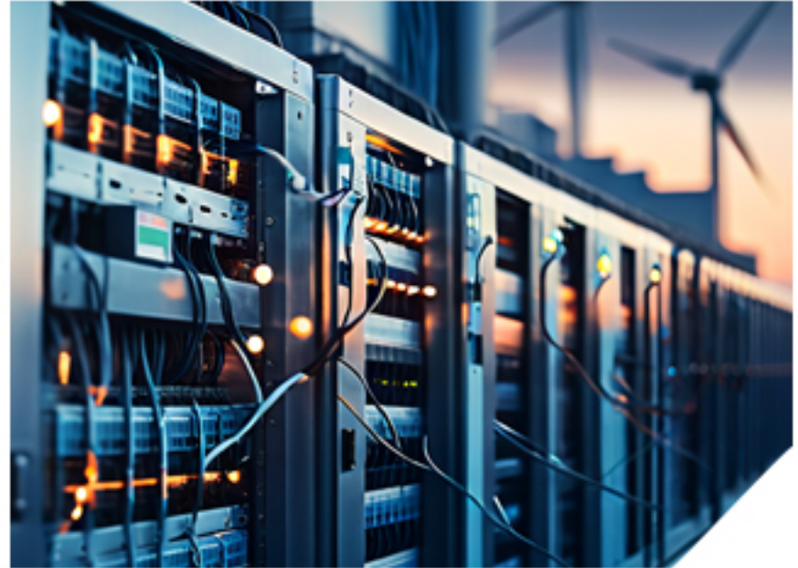
System and Industrial Control Power Supply
